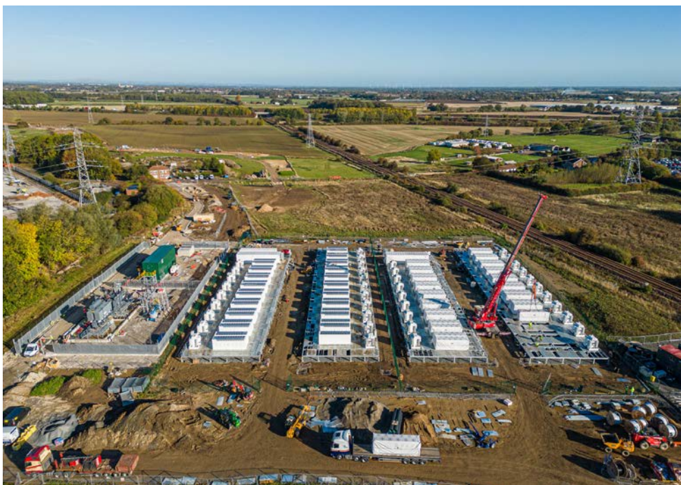
Credit: Harmony Energy
