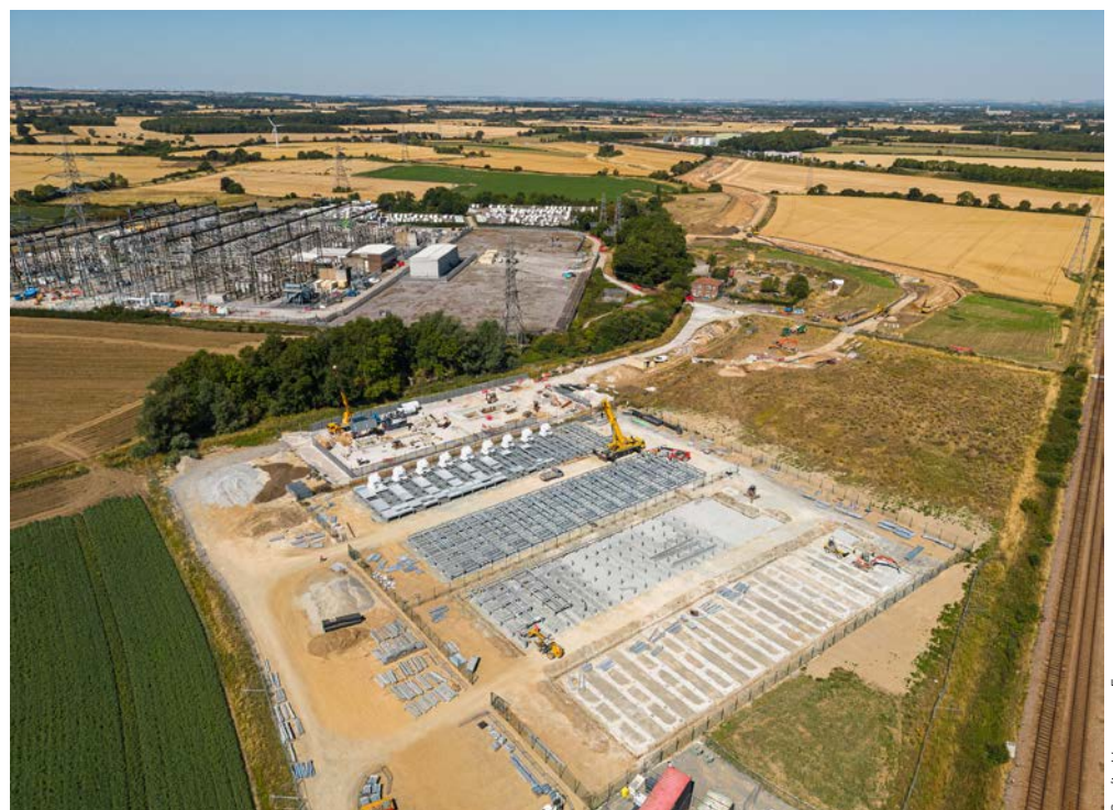
Credit: Harmony Energy.
